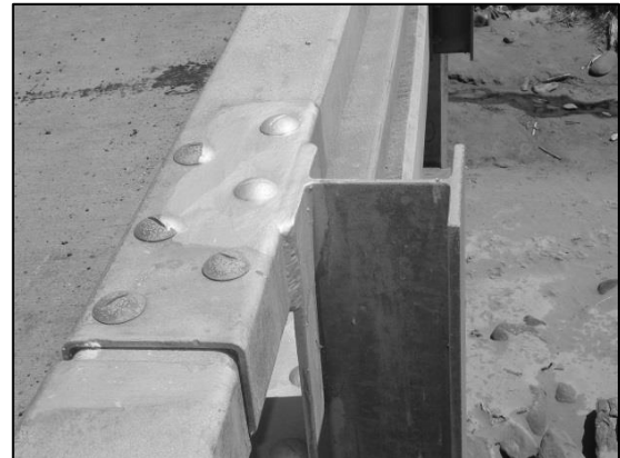
An example of well repaired handrail in a severe corrosive environment (marine).
